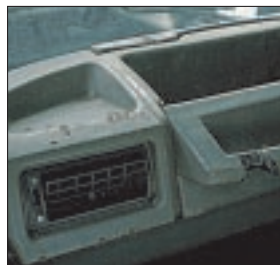
Burns or other damage caused through negligence
