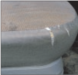
Light surface cracks - due to aging and normal wear
